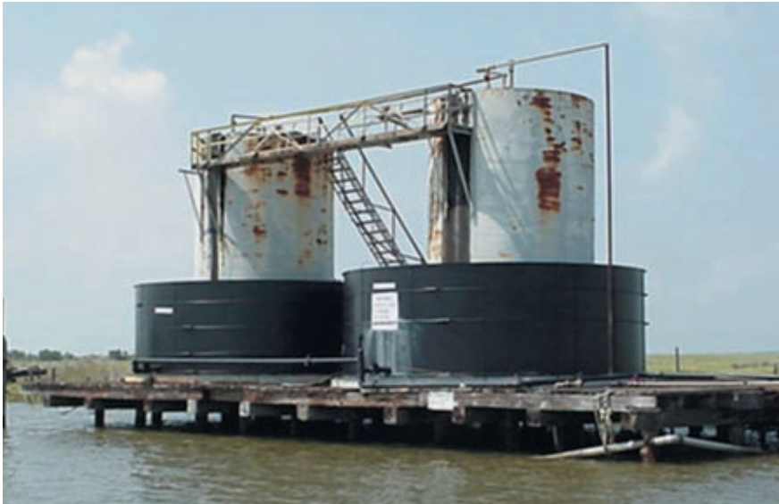
One method of addressing impervious decking requirements is to place existing storage tanks within a larger half tank.
