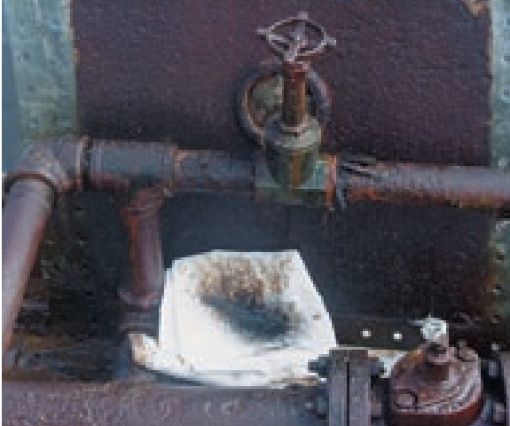
This is not an adequate substitute for a leak-free connection. This leak should be permanently repaired.
