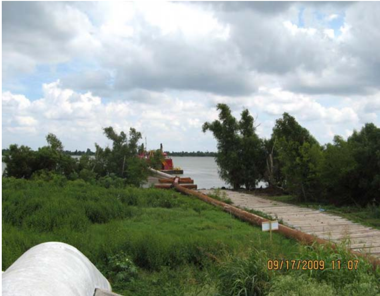
From Booster Pump to Levee
