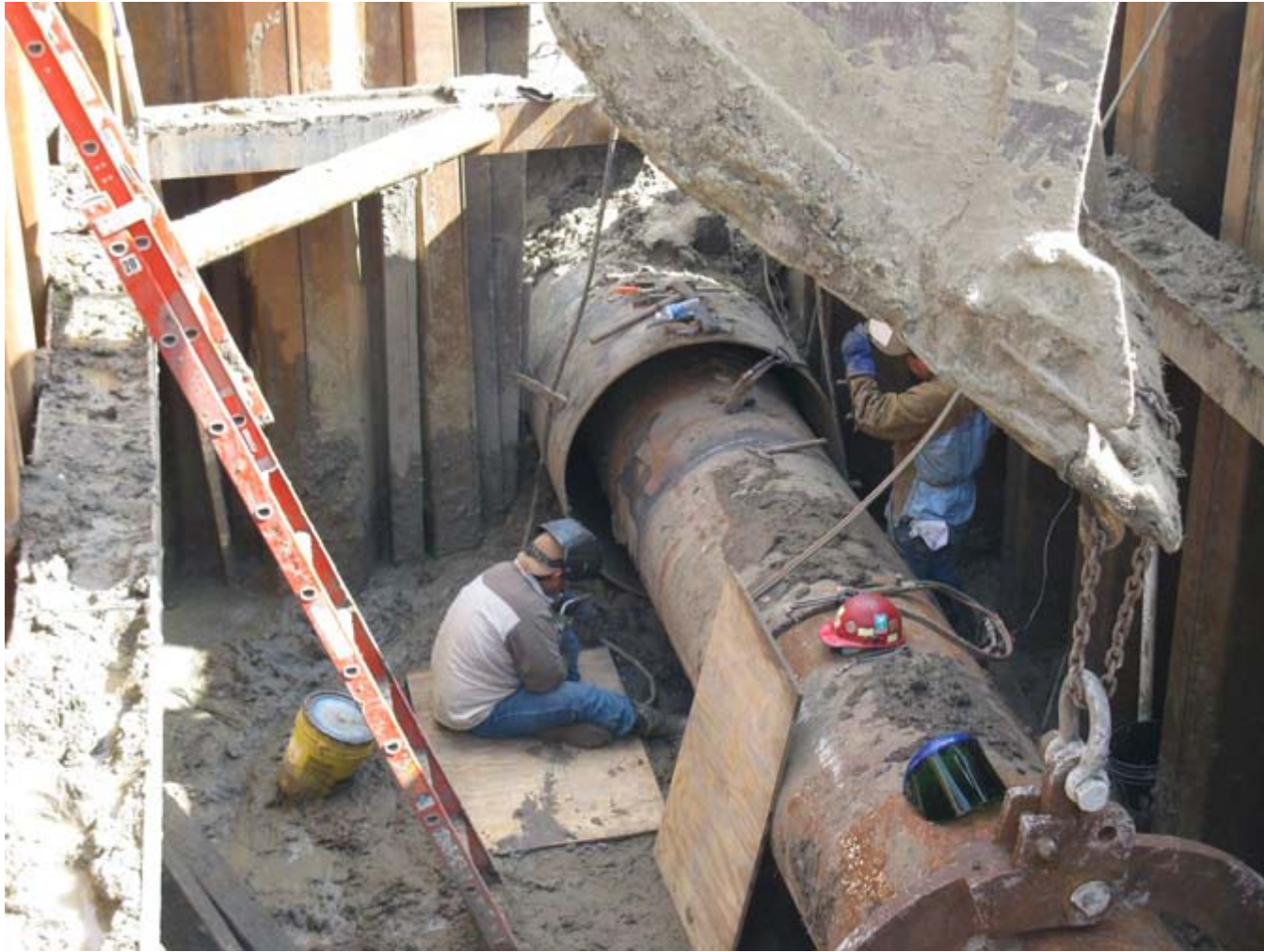
30" dia. Slurry Pipe in 48" dia. Casing
